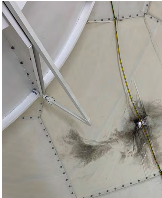
Lightning strike damage to the radar radome.
